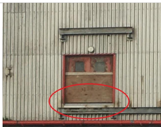
Photo 5. Gap behind plywood (F006) in B4
