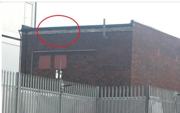
Photo 4. Gap in under bargeboard (F005) in B3
