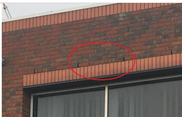
Photo 6. Shallow gaps in brickwork (F007) in B5
